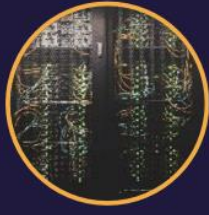
Data centers & Communication networks
